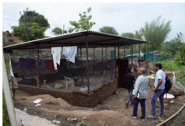
A farmer constructed new goat shed with brick wall & GI sheet roof for keeping goats
